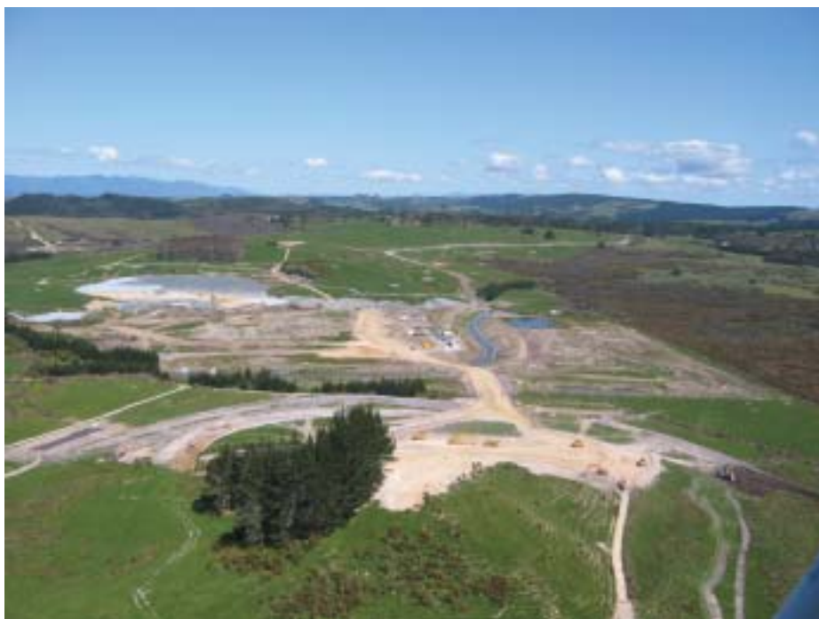
This west facing photo of the new Northland Region Corrections Facility shows the building platform, site sheds and SH12 access road. (Centre right)
