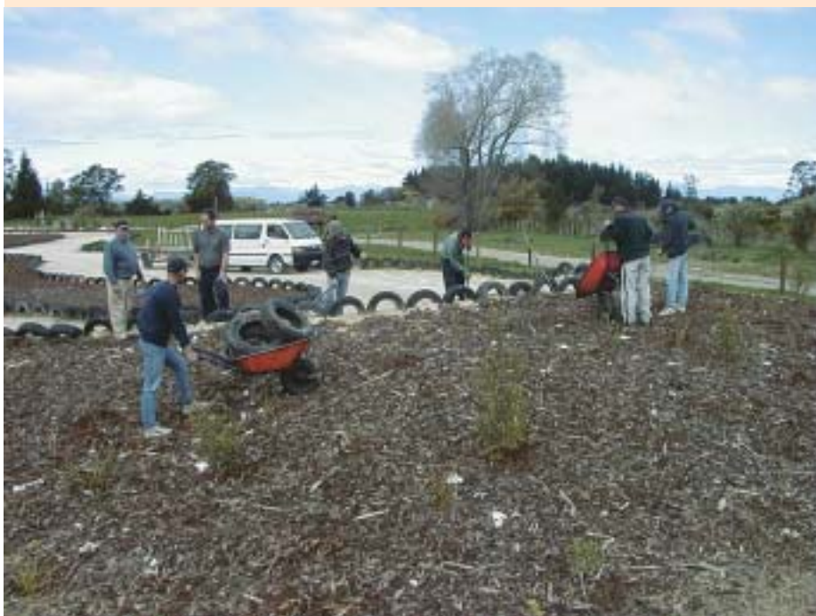
Work party supervisor Graeme Green (far left) oversees work on the go-kart track for the local Cool Kids After School Programme in Motueka.
