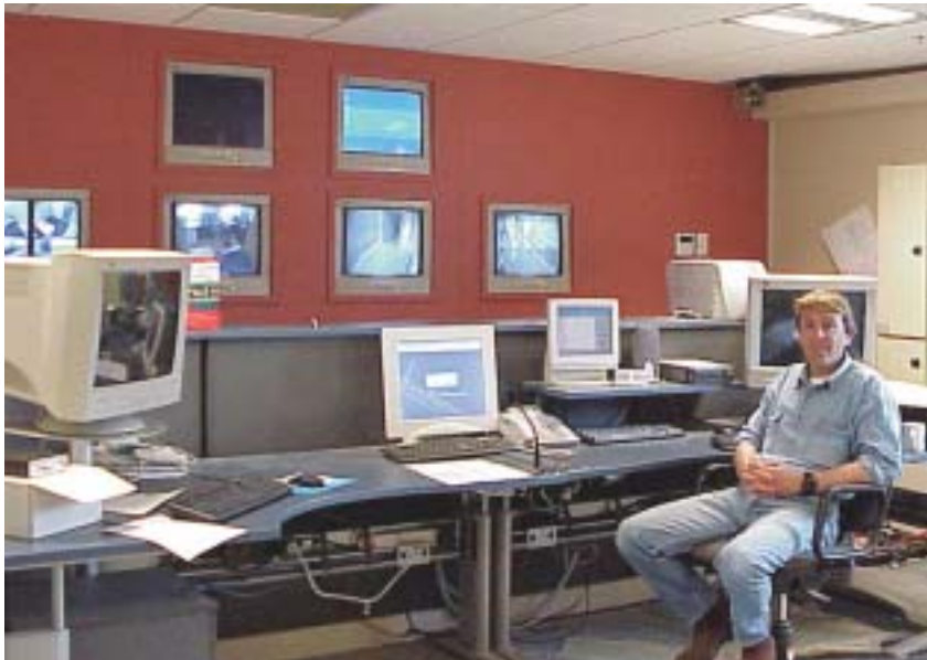
Project Manager Richard Zdrahal in the new movements control room.
