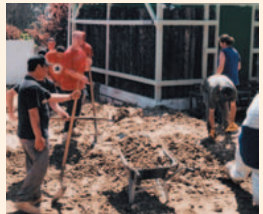
Porirua community workers cleaning up mud and rock at the Belvedere Motel.
