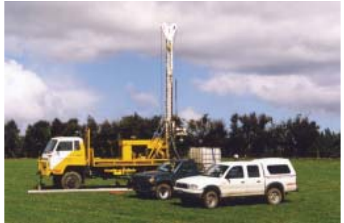
A drill-rig tests the "buildability" of the area on the site at Milburn where the main prison buildings are planned.
